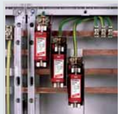
DB NH00 255 H applied in a busbar terminal field of a meter system
