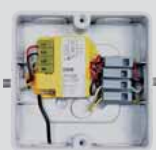
DSM installed into a surface-mounted distribution board
