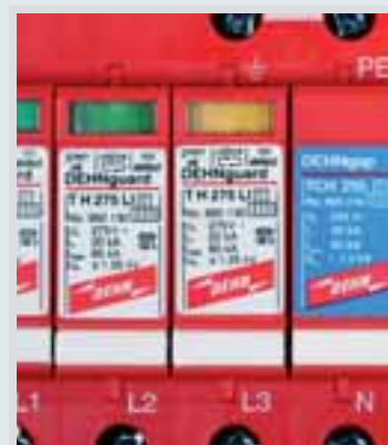
Yellow phase: Replacing of the protection module recommended
